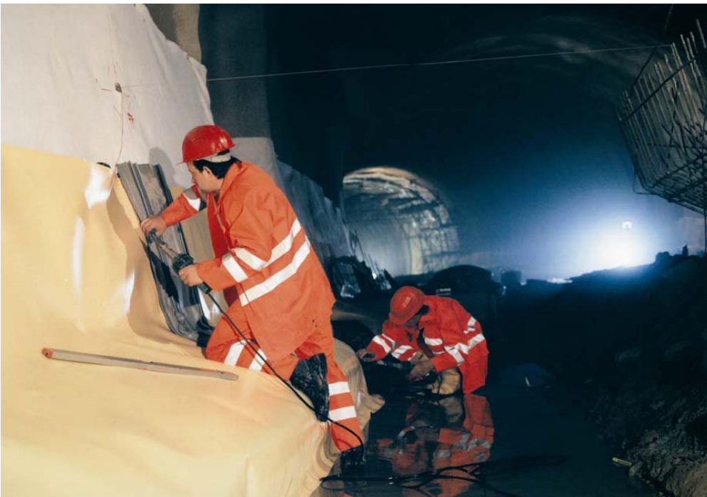
During hot-air welding, working speed and temperature have to be absolutely right. Specially trained membrane welders seal two the overlapping membranes in a double seam.
